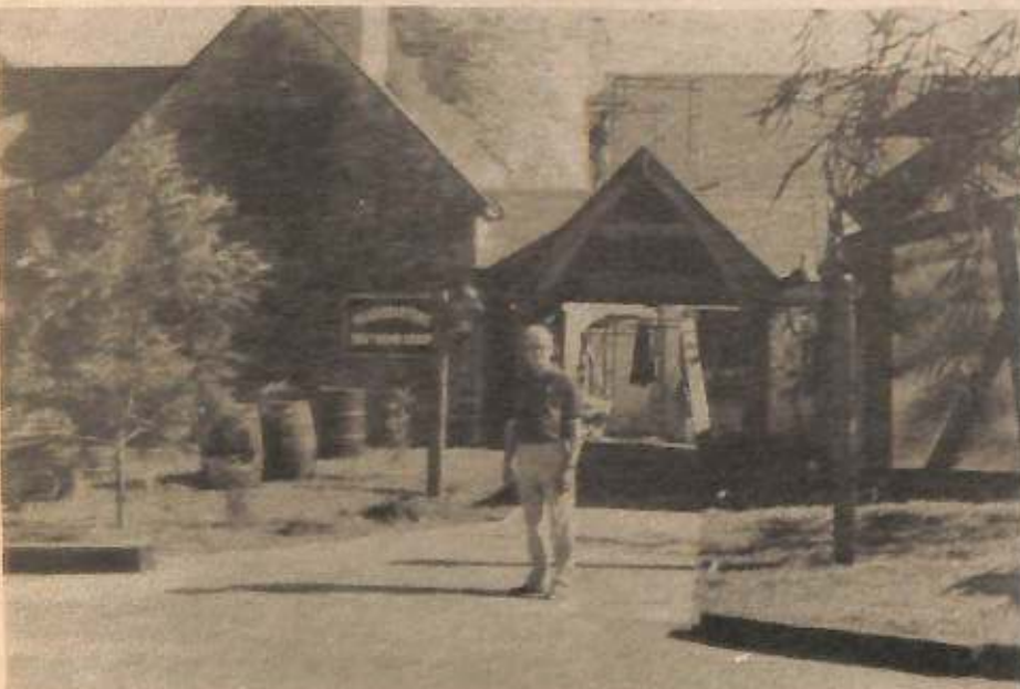
Russell Strong, editor of Echoes, stands outside the uncompleted entrance of the 306th Bomb Group Restaurant. Note the scaffolding in the entry way.
